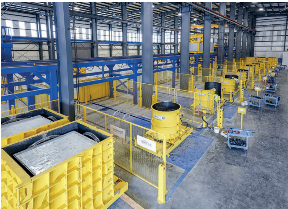
Several set-up locations for wet cast moulds ensure that there are no delays in the overall system despite varying set-up times.
